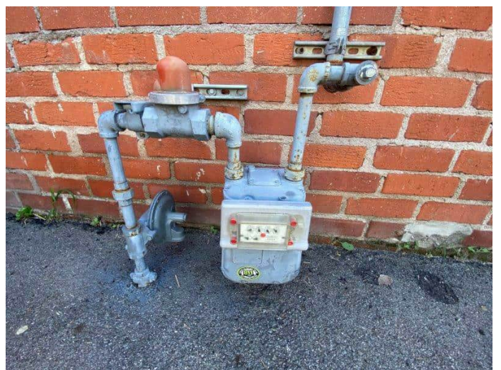
12. Natural gas connection
