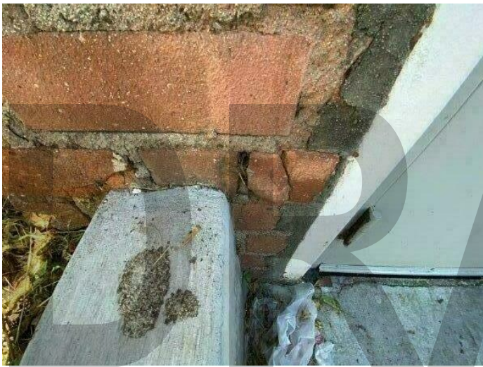
69. Instance of deteriorated mortar at northeast corner of the building
