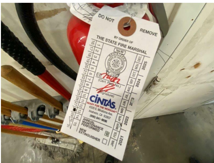
53. Up to date inspection tag on the fire extinguisher
