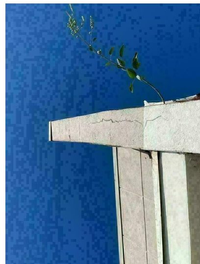
66. Vertical cracking at the southeast corner of the building
