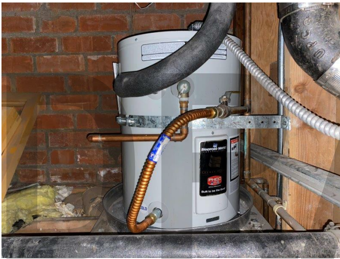
45. Hot water heater note copper supply piping (center/lower right) and cast iron sanitary waste piping (bottom)
