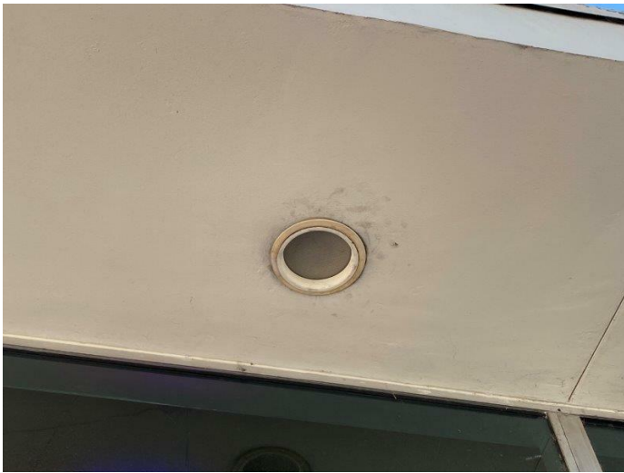
13. Soffit lighting component
