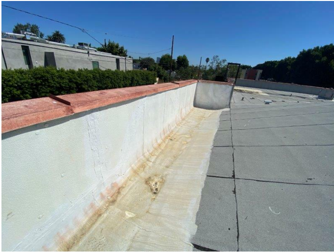
37. Parapet wall and area of recent repair on the northwest corner of the roof
