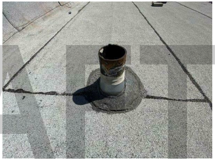
46. Sanitary vent piping
