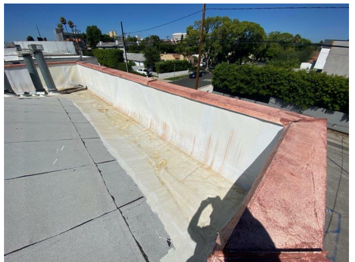
36. Parapet wall and area of recent repair on the northwest corner of the roof
