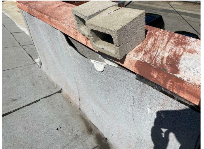
38. Material separation at the inboard side of the parapet wall
