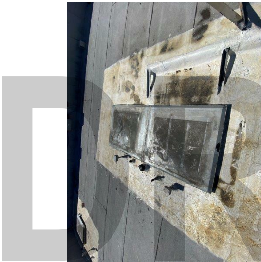
39. Area of removed HVAC equipment and recent roof repair
