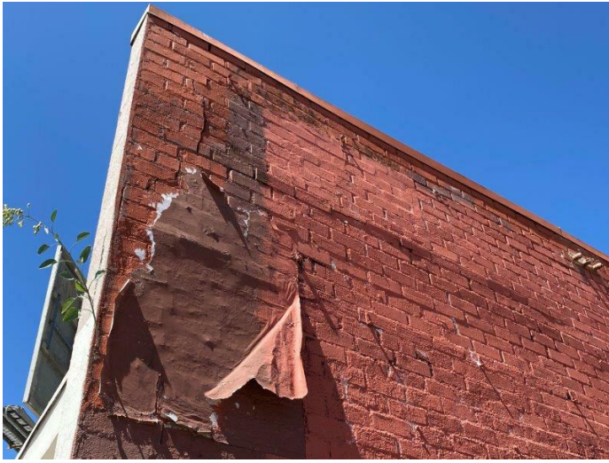
67. Cracking at the southeast corner
