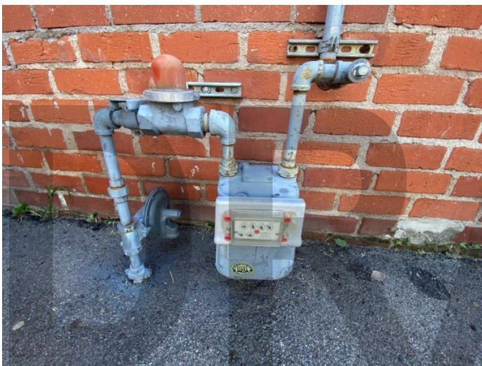
15. Natural gas connection with seismic shut off
