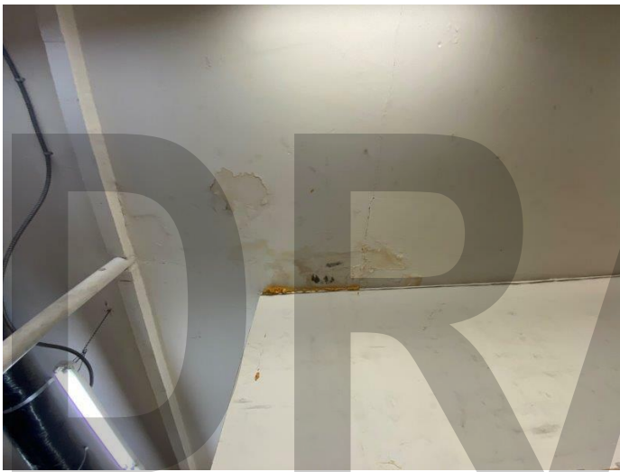
63. Staining at ceiling
