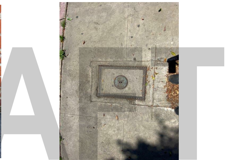
16. Water utility vault in the municipal sidewalk
