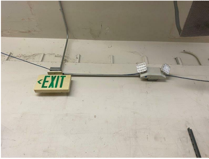
55. Emergency lighting and exit signage
