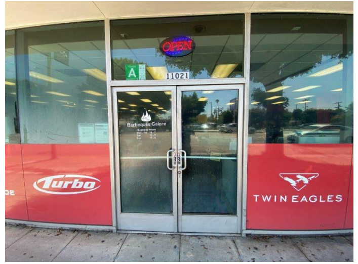
74. Storefront system at the main entrance note address identification signage - note fogged panes at doors and windows
